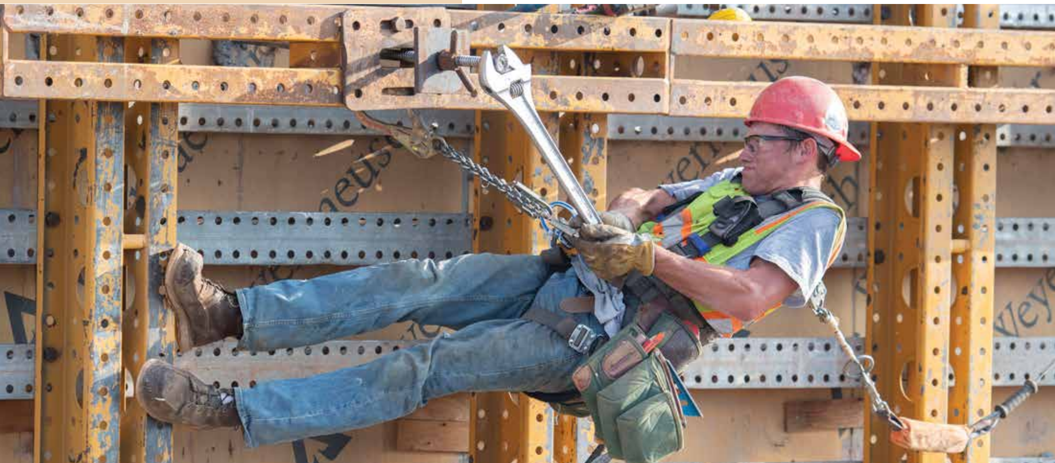
Austin Westling, member of Pile Drivers Local 1847, puts his back (and his entire body) into stripping framework from a cantilever retaining wall on the Gold Line bus route in Maplewood. The Gold Line starts in Woodbury and ends in downtown St. Paul at the Union Depot.
